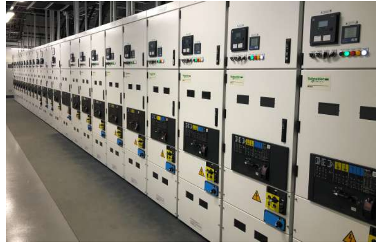
Macquarie Data Centres, compliant with the IEC-61850-3 standard, mitigates interoperability issues while integrating advanced technology between systems.
